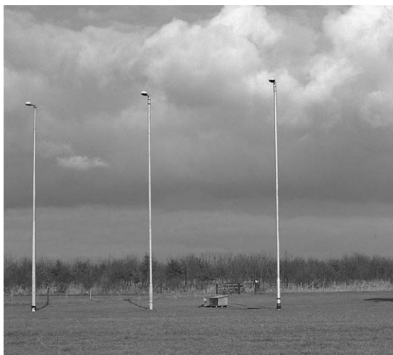
Fig. 2. Experimental lighting columns at the SRI test site.
