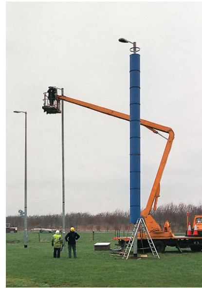
Fig. 5. Plastic drums used to enlarge the diameter of one of the lighting columns.
