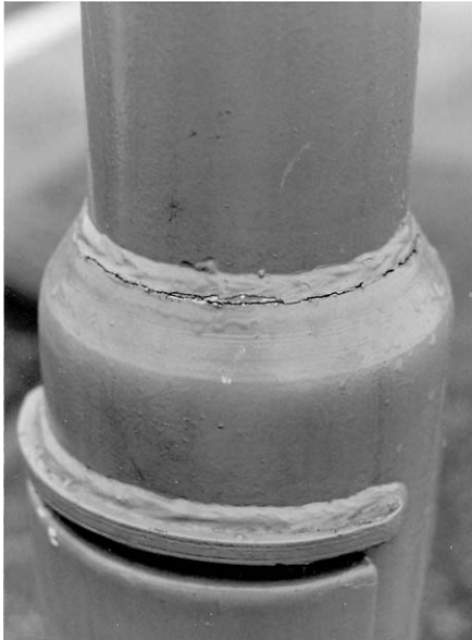
Fig. 1. Fatigue crack in a lighting column in service.
